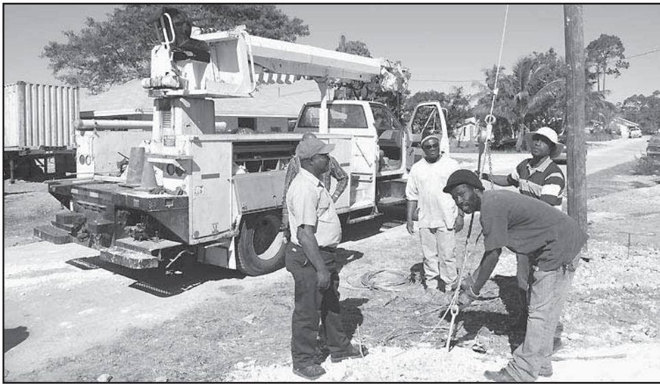
While the Minister of Housing, the Hon. Kenneth Russell, was inspecting the construction of government built houses in Spring City, a BEC crew was extending the electric lines to the houses almost completed.
