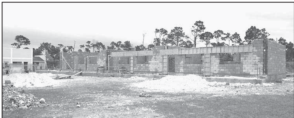
The second building is a block with three classrooms for technical training. This construction is being done by Williams & Sons Construction Co. Ltd. It will include rest rooms and is expected to be completed by the end of the year.
